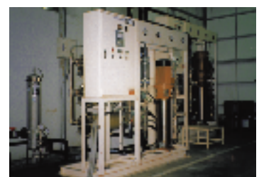
Waste water Recycling system Recycles a total of 150 tons a day.
