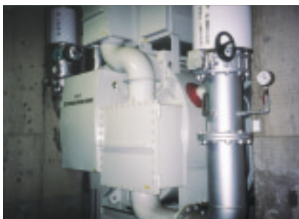
Cool and warm water generating system
