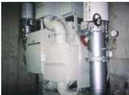
Cool and warm water generating system
