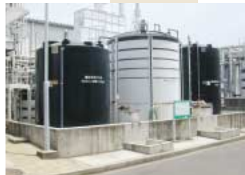
Leakage Containment Barrier
