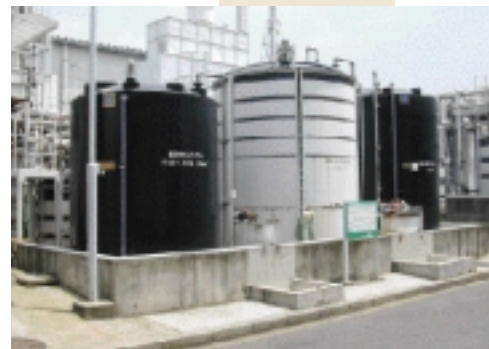
Leakage Containment Barrier
