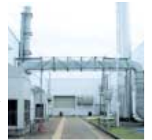
▲Duct Used for Discharging Heat from the Machine Room
