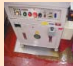
Oil trays installed under machinery
