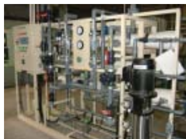
RO condensate return equipment, which generates highly purified water
