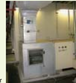
Outdoor air conditioner
